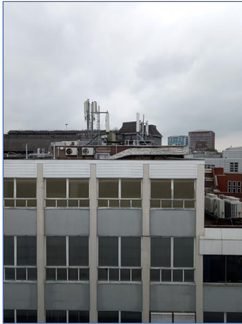
Fig 1. Existing rooftop equipment to 41 Minster Street as viewed from the roof of Holy Brook Car Park.
