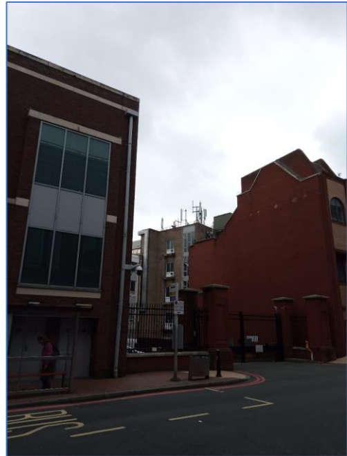
Fig 2. Existing rooftop equipment to 41 Minster Street as viewed from ground level on Minster Street.
